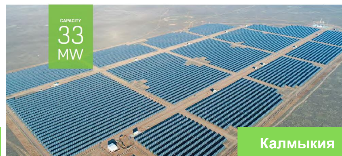
Yashkul Solar Power Plant, Republic of Kalmykia
